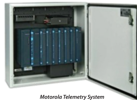
Motorola Telemetry System
